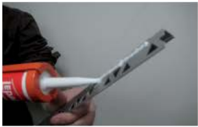
Add adhesive caulking on the rear of the ARTOTRIM-L1 trim and affix to the wall.
