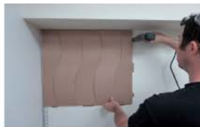
Put the first tile on the ARTOTRIM-L1, staple all the visible tabs on the tile. Make sure the tiles are aligned.
