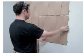
Continue the installation and verify the tile alignment using the reference line or laser for a symmetrical finish.
